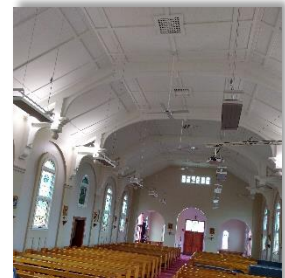
ST. JOSEPHS PARISH EXISTING PANEL HEATERS
