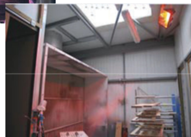
Wood works Paint Booth
